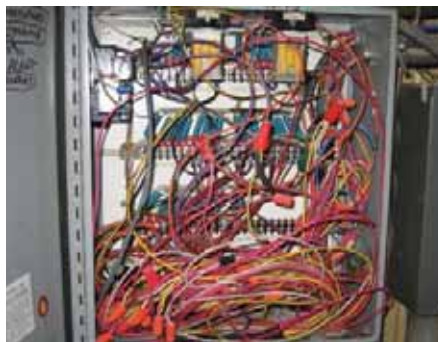
An example of a wiring junction box that has been modified over the years.
